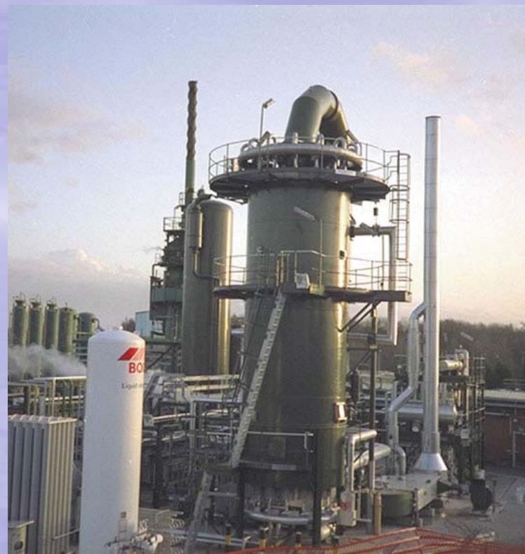
Hydrogen plant supplied to BOC St. Helens, England
